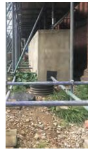
The temporary works structure was ballasted by concrete kentledge blocks, buried up to 2m in the ground
